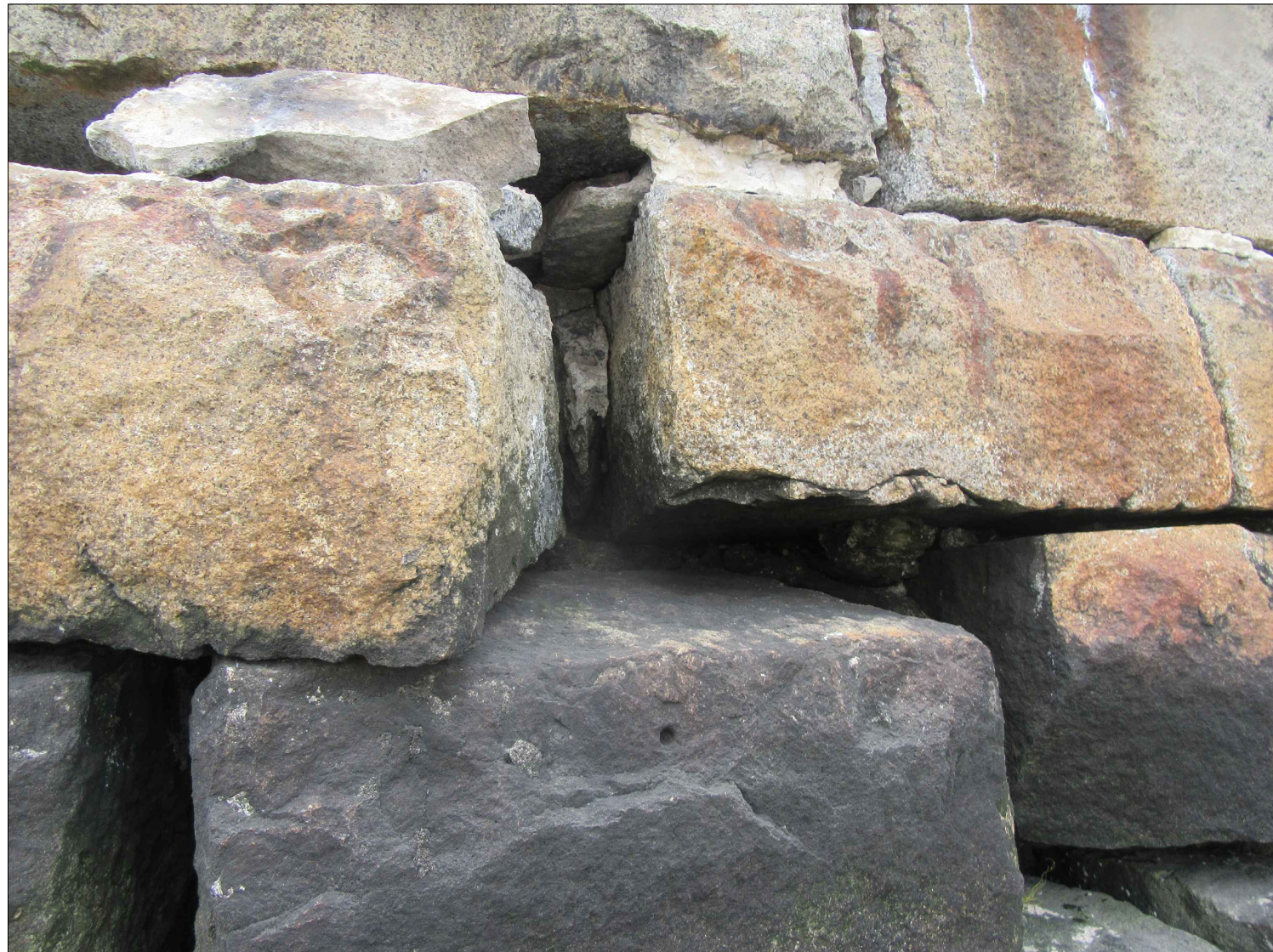
PHOTO 4: CORNER OF SOUTH AND EAST SEAWALL, HIGH TIDE
