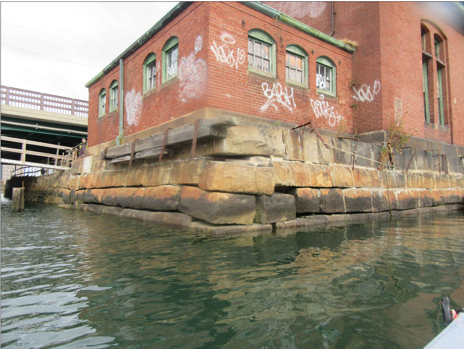
PHOTO 5: SPACE BETWEEN GRANITE BLOCKS AT CORNER OF SOUTH AND EAST SEAWALL
