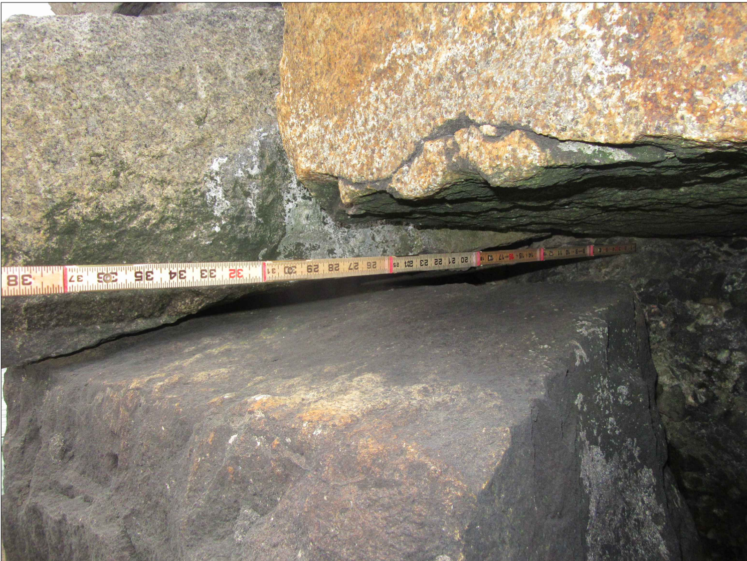
PHOTO 6: ENLARGED VIEW OF TYPICAL JOINT BEARING LOSS AT CORNER OF SOUTH AND EAST SEAWALL
