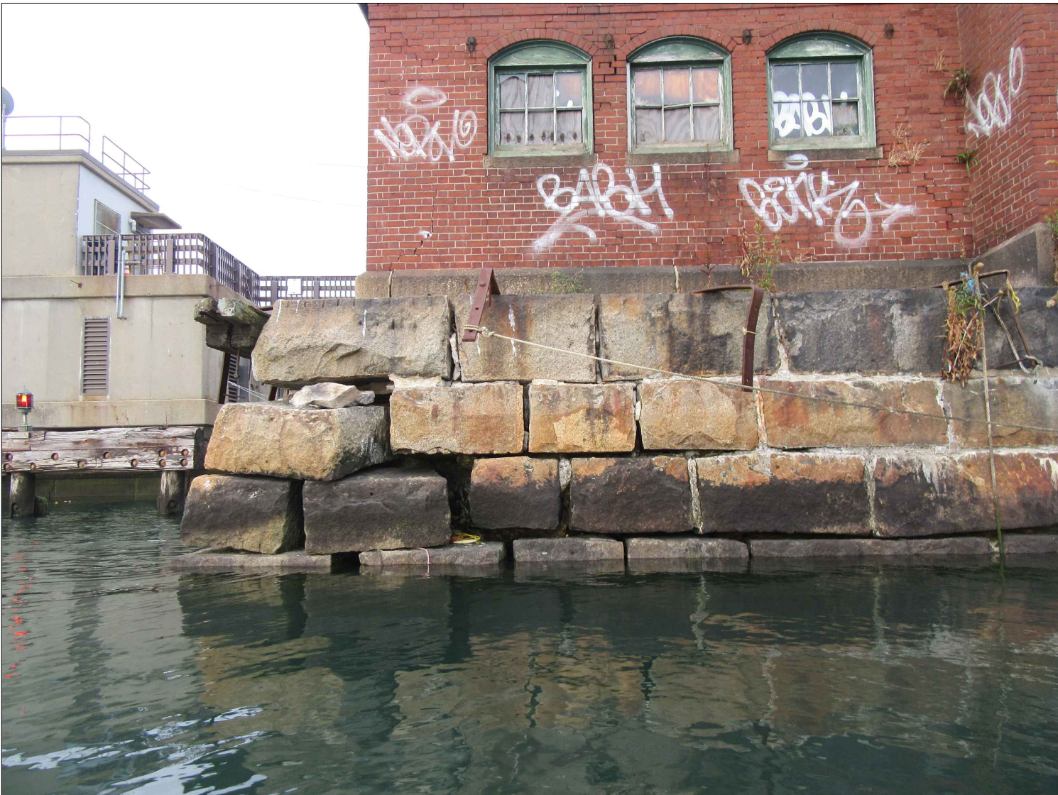
PHOTO 3 : EAST SEAWALL, HIGH TIDE CLOSE UP OF SHIFTED GRANITE BLOCKS AT CORNER
